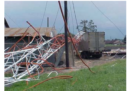
Communications Tower destroyed in Mississippi
